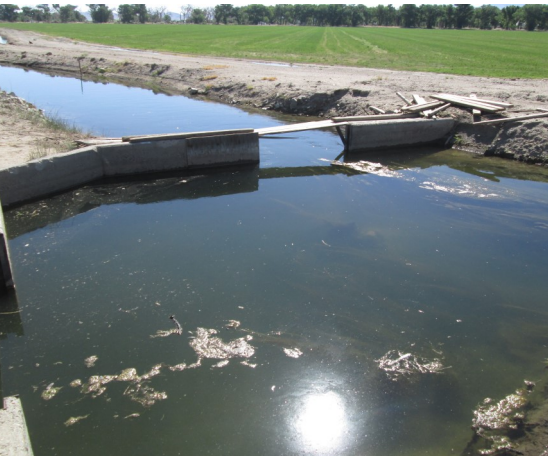
Campbell Canal Split Structure
